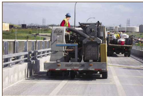
Automatic Shot Blasting Equipment Used to Prepare the Deck Panels for the Overlay
